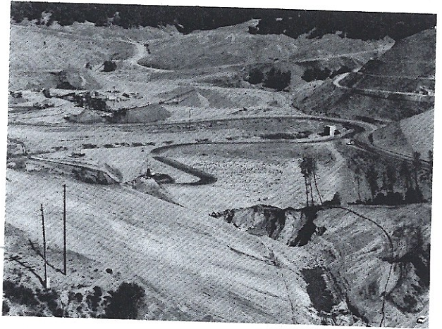
The spillway and entrance to the fish ladder are still under construction.
